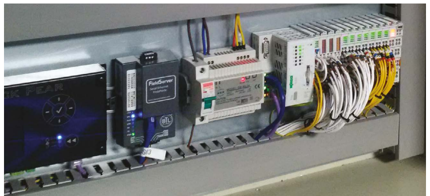
WAGO-I/O-SYSTEM 750 modules were used to provide heating and lighting controls.
